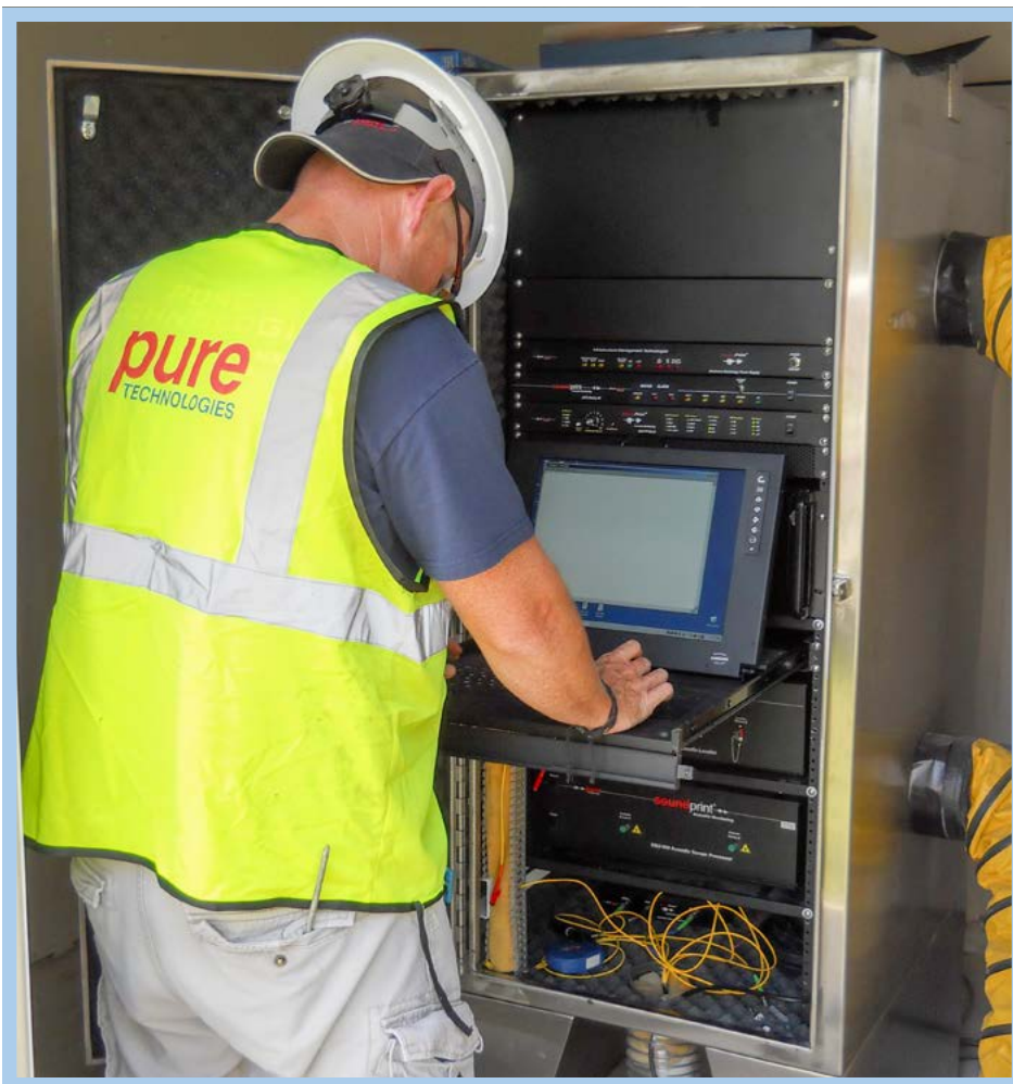
AFO Data Acquisition System located at the SPS.
