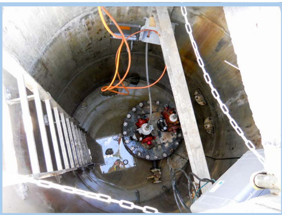
Below: Typical AFO Splice Box and entry and exit point at an SRFM Inspection Manhole.
